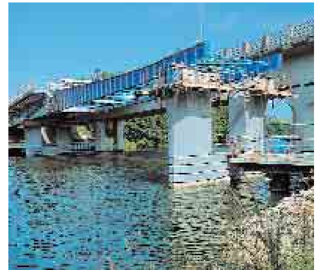
For Jonches bridge, 'we wanted to demonstrate that we could use HPC to construct a bridge at a cost equivalent to the cost of a steel bridge'.
