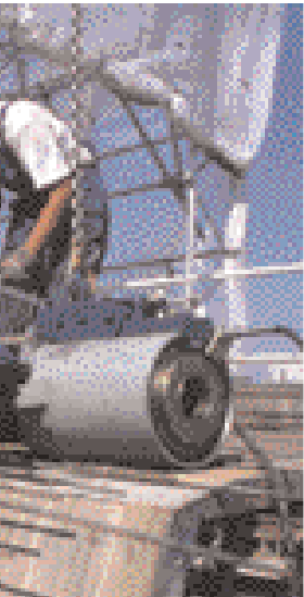
Two parallel decks form the Czerniakowski interchange. They are built using the incremental launching method.
